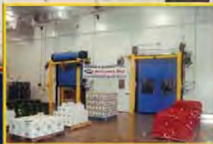
42,000 SQUARE FEET OF REFRIGERATED SPACE
